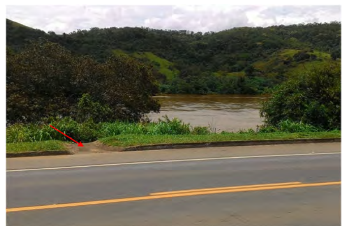
Fig. 4. Section of the Lúcio Meira highway (BR-393) with a surface drain (red arrow) into the Paraíba do Sul River, in southeastern Brazil.
